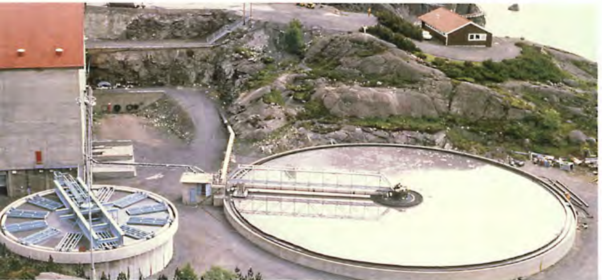
Installation of a Svedala LTC Combi lamella clarifier next to a conventional round thickener with approximately the same clarification area.
