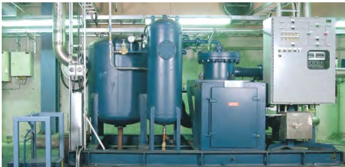
SVEDALA HGMF used in a stainless steel rolling mill
