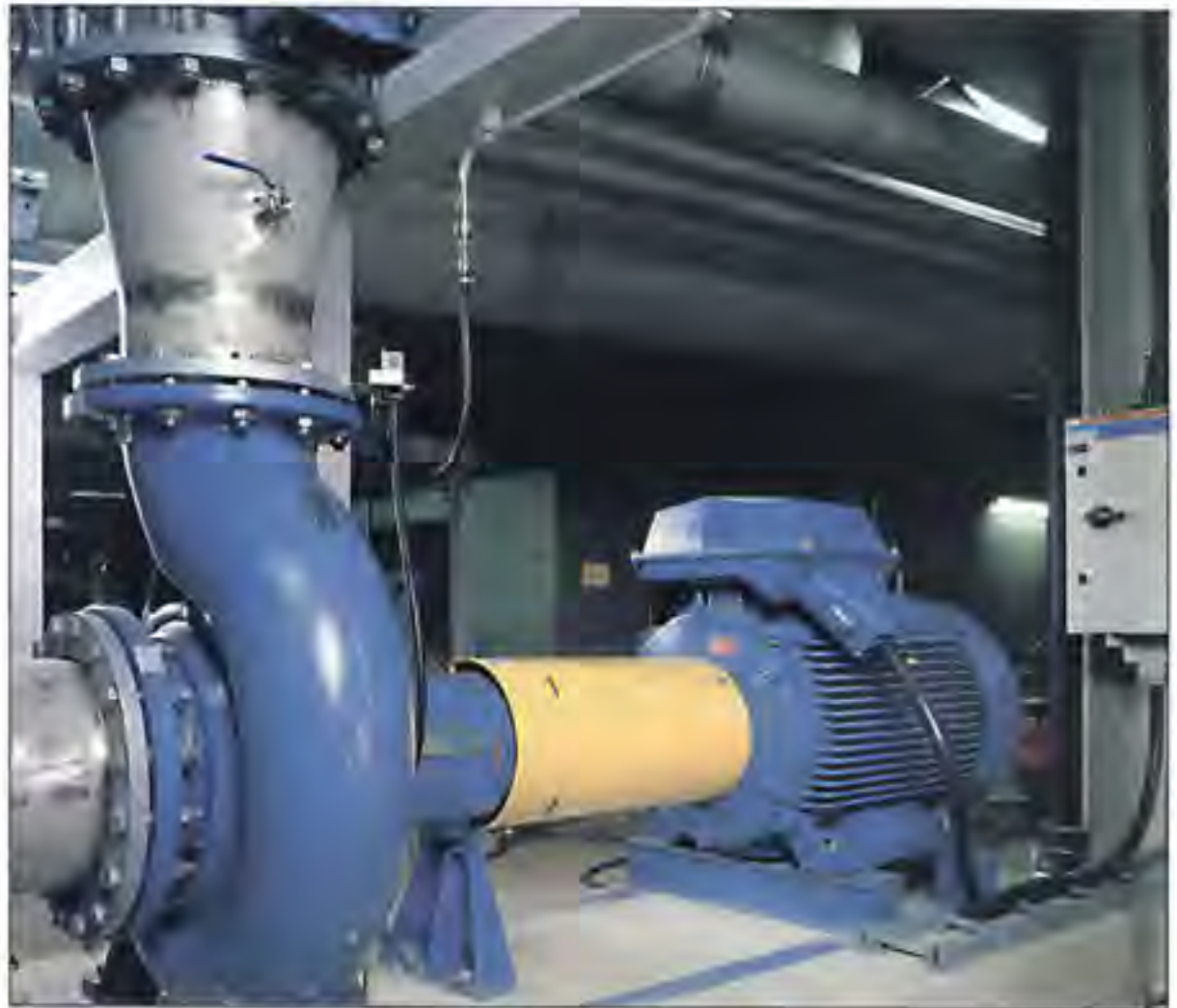
BA 14x12-17 installed in a paper mill pumping paper stock.
