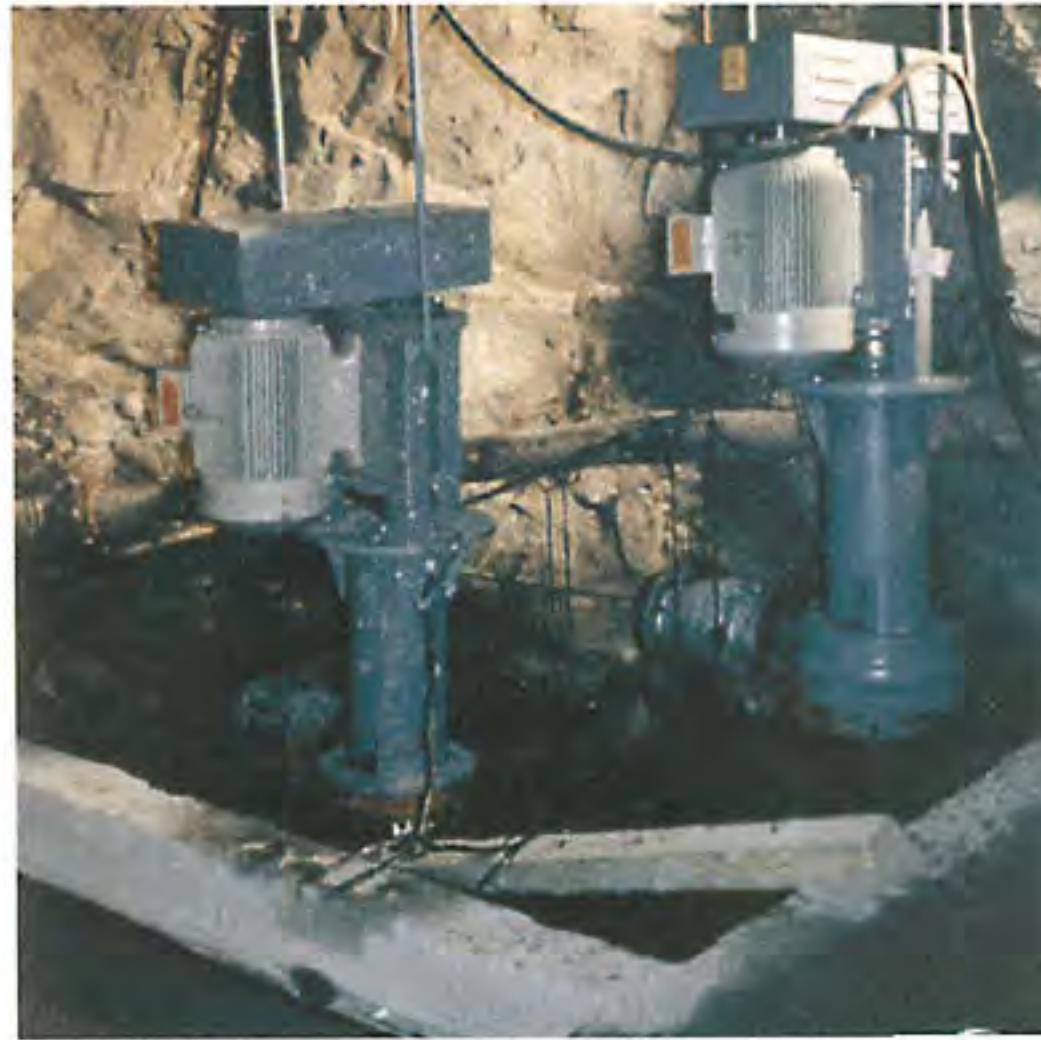
VS100-L120 pumps on a tunnel dewatering service.
